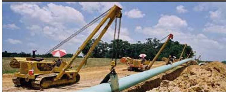
Moheshkhali Gas Transmission Pipeline
